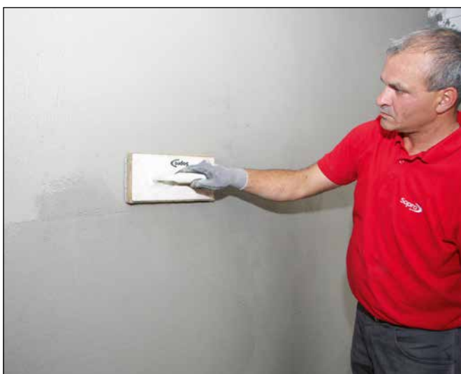
11 Neatly ruled-off render is ready for tiling after 6 hours. If a tile finish is not required, Sopro RAP 2 434 can be additionally rubbed down with a slightly damp sponge float ...
