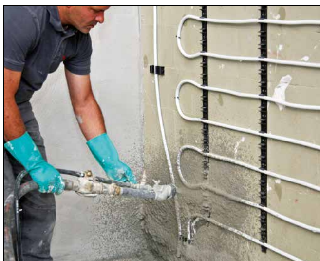
10 Spray application of Sopro RAP 2 434 is also possible for larger areas, as in pictured example, where render is used to embed (Kermi x-net c21) wall heating system.
