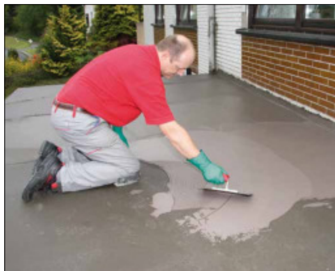
14 Apply second coat when first waterproofing coat has fully dried (after only 2 hours) ...
