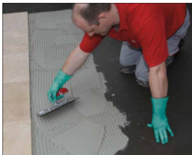
16 Apply two-component Sopro MEG 665 megaFlex S2 or Sopro MEG 666 megaFlex S2 turbo highly flexible tile adhesive to fully cured waterproof membrane.
