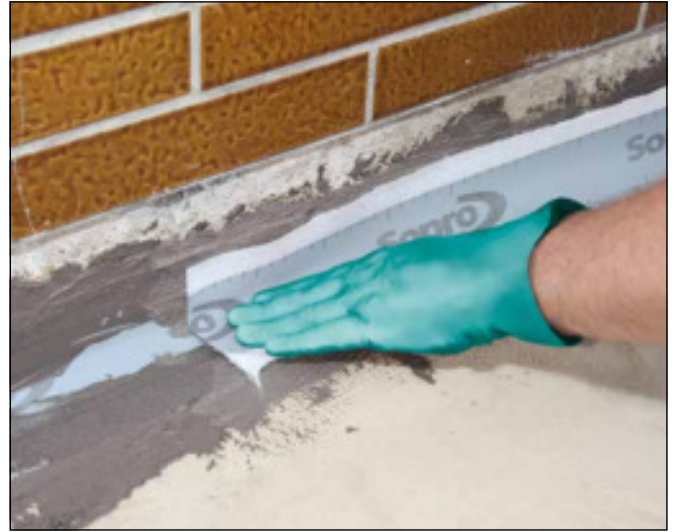
8 ... subsequent placing and fixing of Sopro DB 438 sealing tape. Ensure that tape is firmly pressed down.
