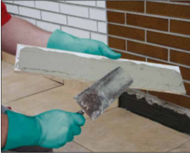
19 Apply Sopro flexible adhesive (e.g. Sopro's No.1 400 or Sopro FKM XL 444) to rear face of cut-to-size skirting tiles ...
