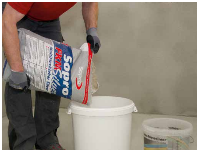
1 Mixing of Sopro FKM 600 to required consistency for thin-bed, floating-bed or medium-bed laying or for surface filling.
