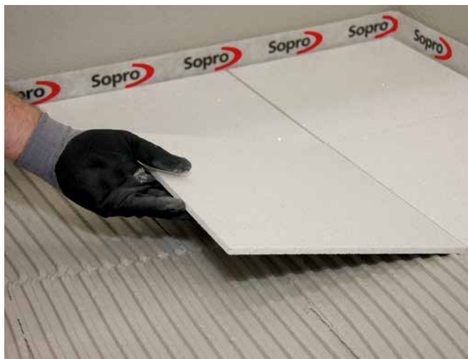
2 Laying of agglomerate tile. Rapid-set properties of Sopro FKM 600 also make it suitable for laying deformation-sensitive coverings.
