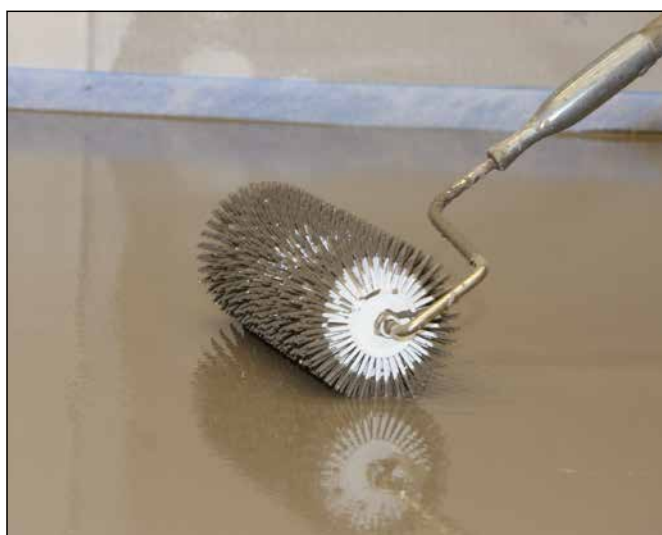
9 A spiked roller may be used to release entrapped air from applied filler compound.
