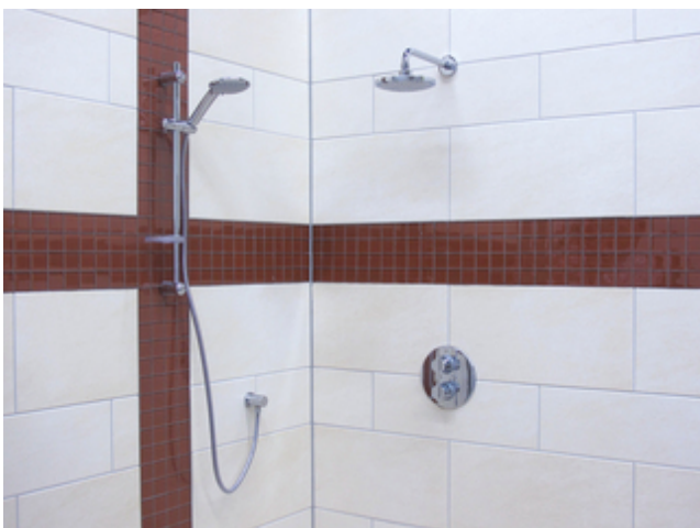
11 Brilliantly coloured joint surfaces in bathroom.
