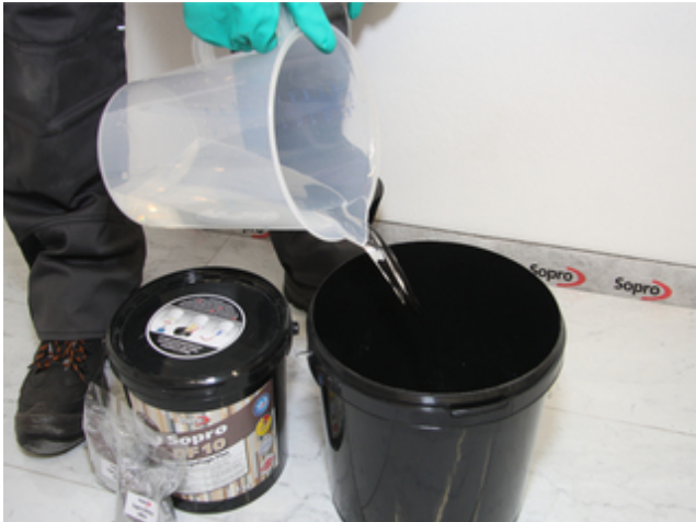
1 Fill clean bucket with clean mains water.
